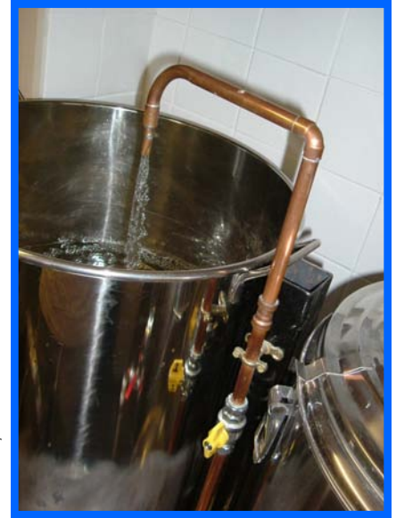
Spraying brewing liquor into the Hot Liquor Tank.
